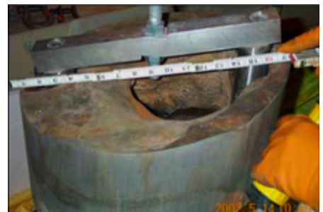
Erosion of the 150-millimetre-thick (5.9 in) carbon steel reactor head at Davis-Besse Nuclear Power Plant , in Oak Harbor, Ohio, USA , in 2002, caused by a persistent leak of borated water .
